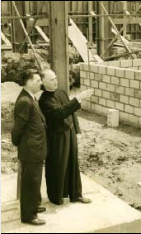
Fred Jacques '34 inspects construction on the Kennedy (formerly Hudson) Boulevard campus with Father James J. Shanahan, S.J., in the 1950s. Jacques served at the College for more than 40 years as a Chemistry professor and alumni director.
